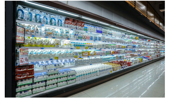
S-store /C-store /supermarket Area: 300m 2 -2000m 2 Cabinet Temp.: -1°C ~ +10°C OAT: -30°C ~ +48°C
